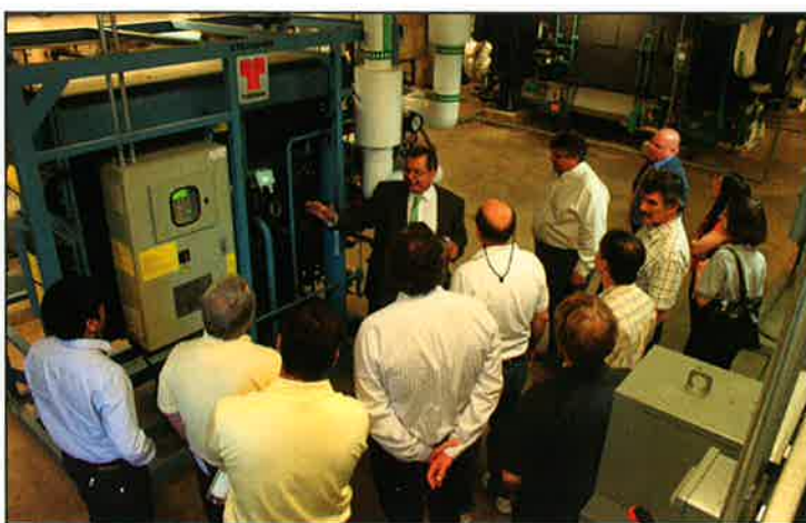
Sherif Youssef, director of sales & marketing, explaining to PGW's guests the benefits of using the waste heat in the summer to run a 40 ton Thermamax absorber.
